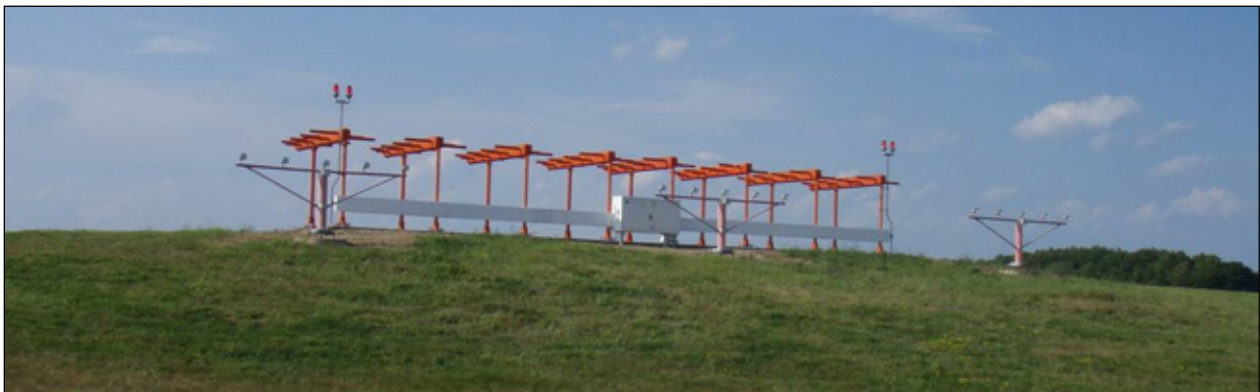
Figure 6-21. LOC 8-antenna array
