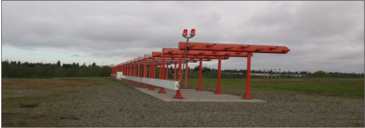
Figure 6-22. LOC 14-antenna array
