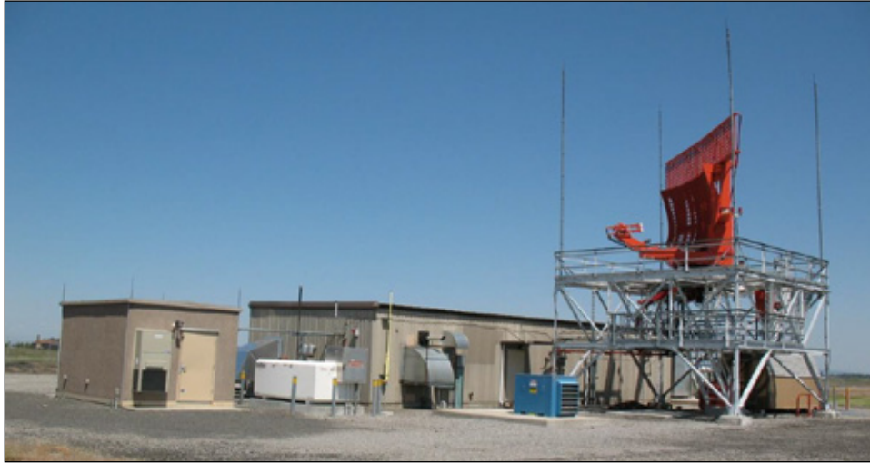
Figure 6-5. Airport Surveillance Radar (ASR) steel tower (17 feet [5 m] high)
