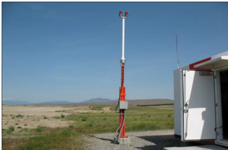
Figure 6-25. Distance Measuring Equipment (DME) antenna
